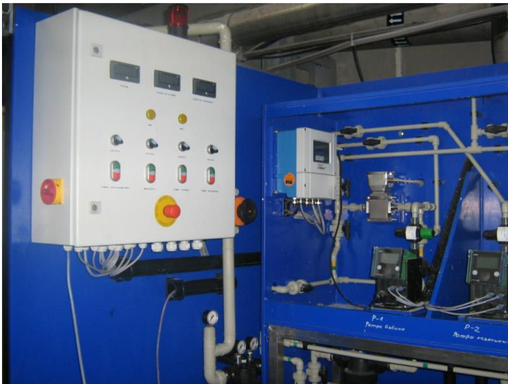
Picture 3. Installed control panel
