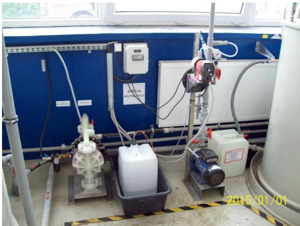
Picture 4. The supplied station for neutralization
