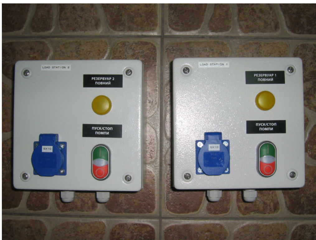
Picture 3. Control panels for filling the storage tanks.
